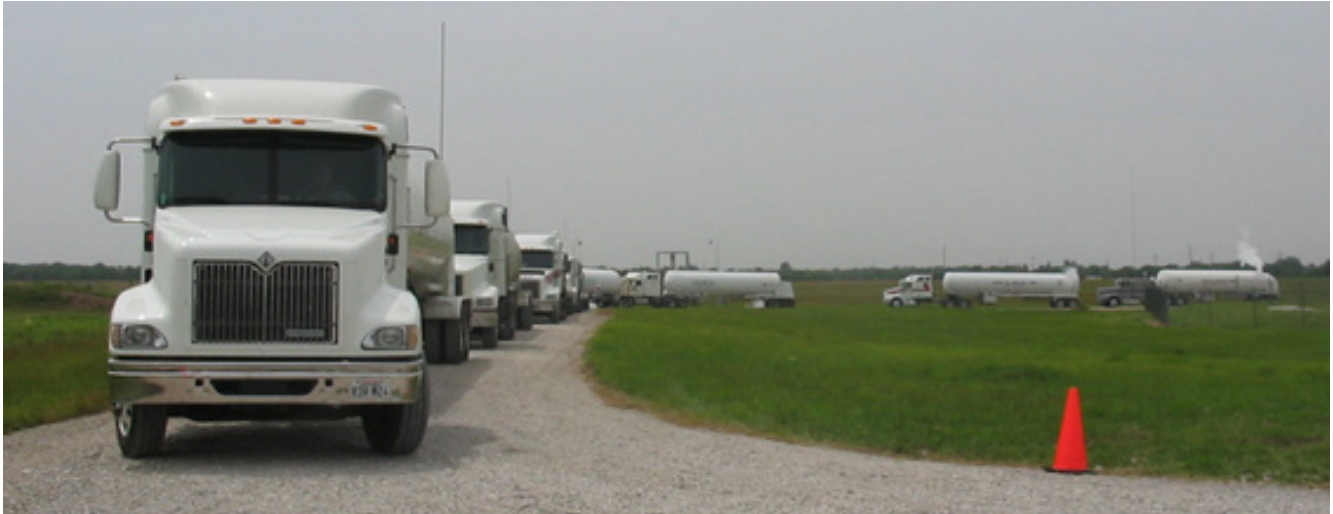
Cryogenic nitrogen transports lined up to support the purge of a 600-mile long 24-inch diameter pipeline.
