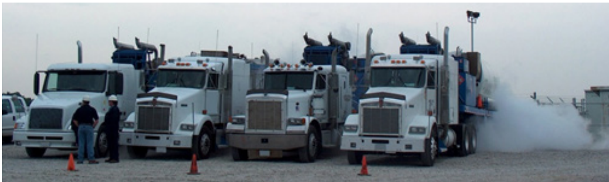
Four Nitrogen Pumpers in operation on the purge of a 600-mile long 24-inch diameter pipeline.
